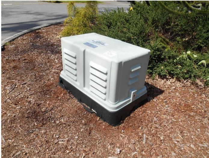
Figure 3 - Example of an Autoflush location
